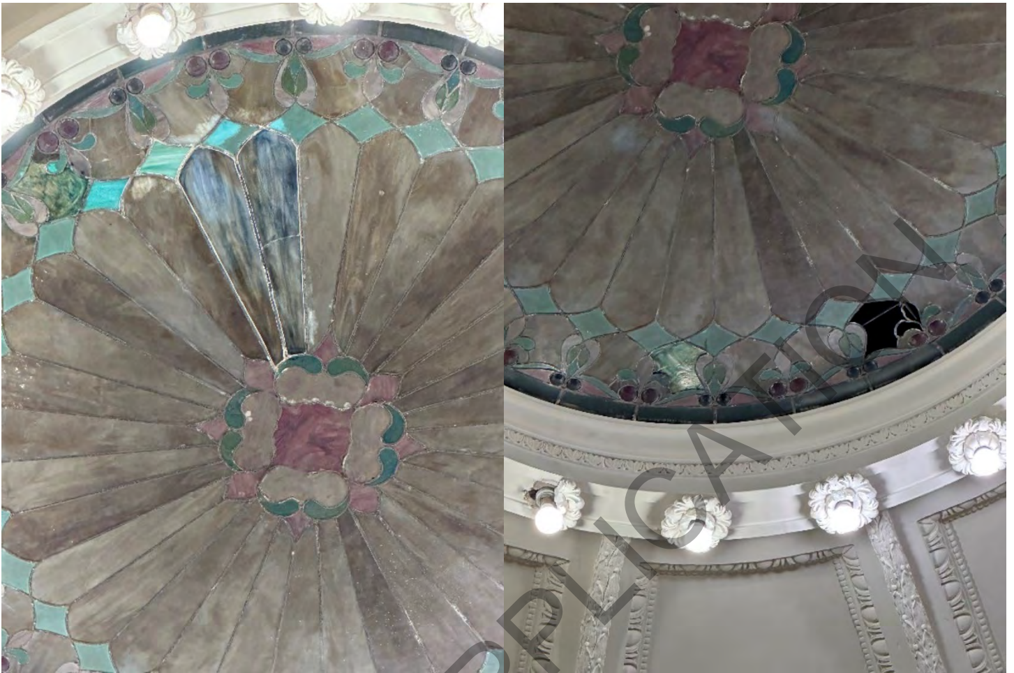
Third floor of the Bataan Building Image 39 (above, left) – Looking up to Rosette window Image 40 (above, right) – Detail of Rosette window
