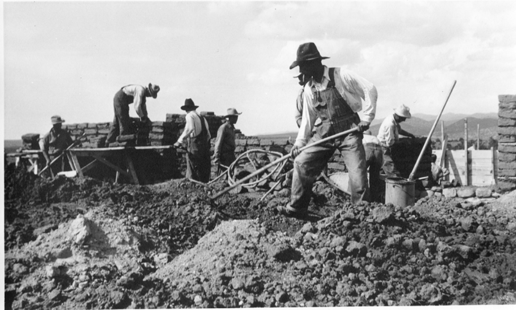
Figure 1. McKibbin House under construction with workers making adobe bricks and using them to form walls
